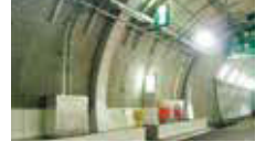
Attachment in the tunnel of capital expressway
