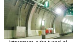
Attachment in the tunnel of capital expressway
