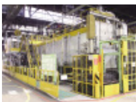
Newly set heat treatment furnace (NH-12 Furnace)
